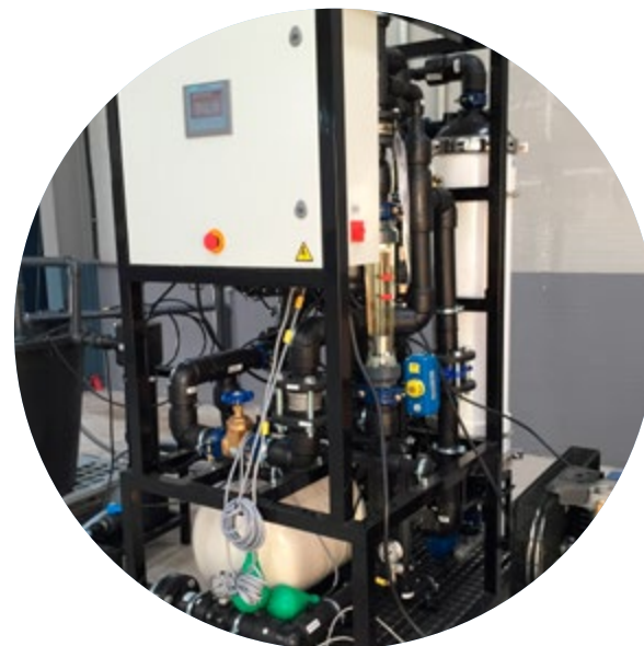
Spain Almería. Vegetables washing process 2 m 3 /h (1 unit)
