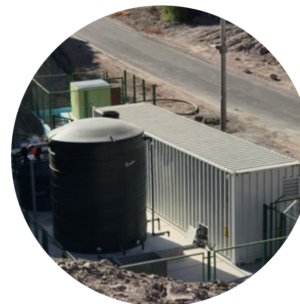
Peru Ilabaya Arsenic and boron removal 6.5 m 3 /h (1 unit)
