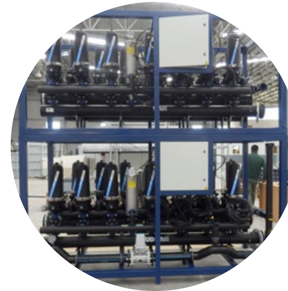
Dubai District cooling plant (3) Conditioning circuit 225 m 3 /h (4 units)
