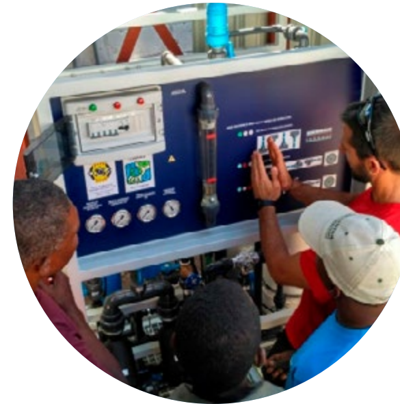
Haiti NGO Matthew storm response operation 3 m 3 /h (2 units)
